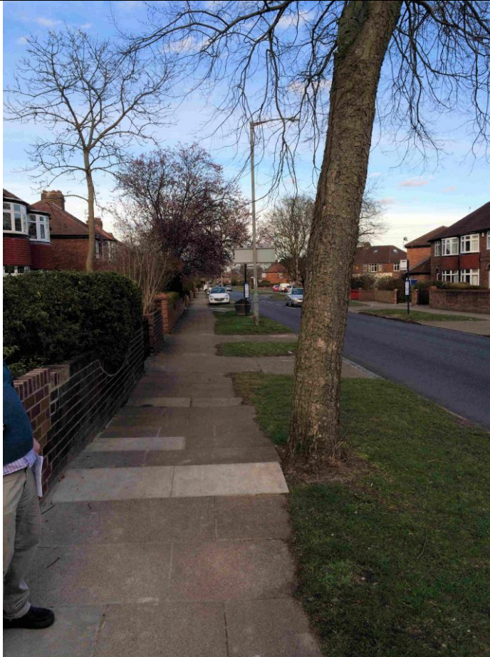
Tree on 248 Hamilton West Drive damaging footpath (above)
